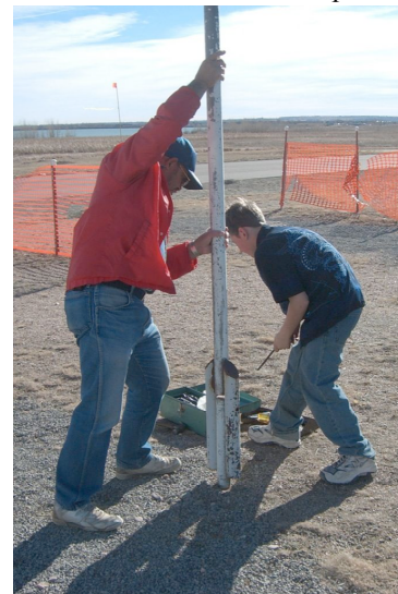
Rudy Furman and Thomas Rooney installing a new windsock at Chandler Field.
